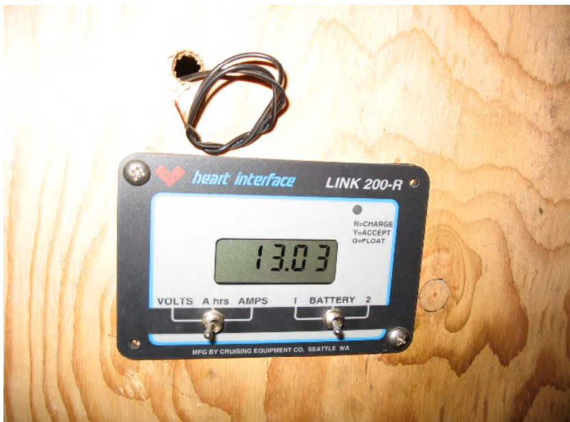
Control and Monitor panel.
